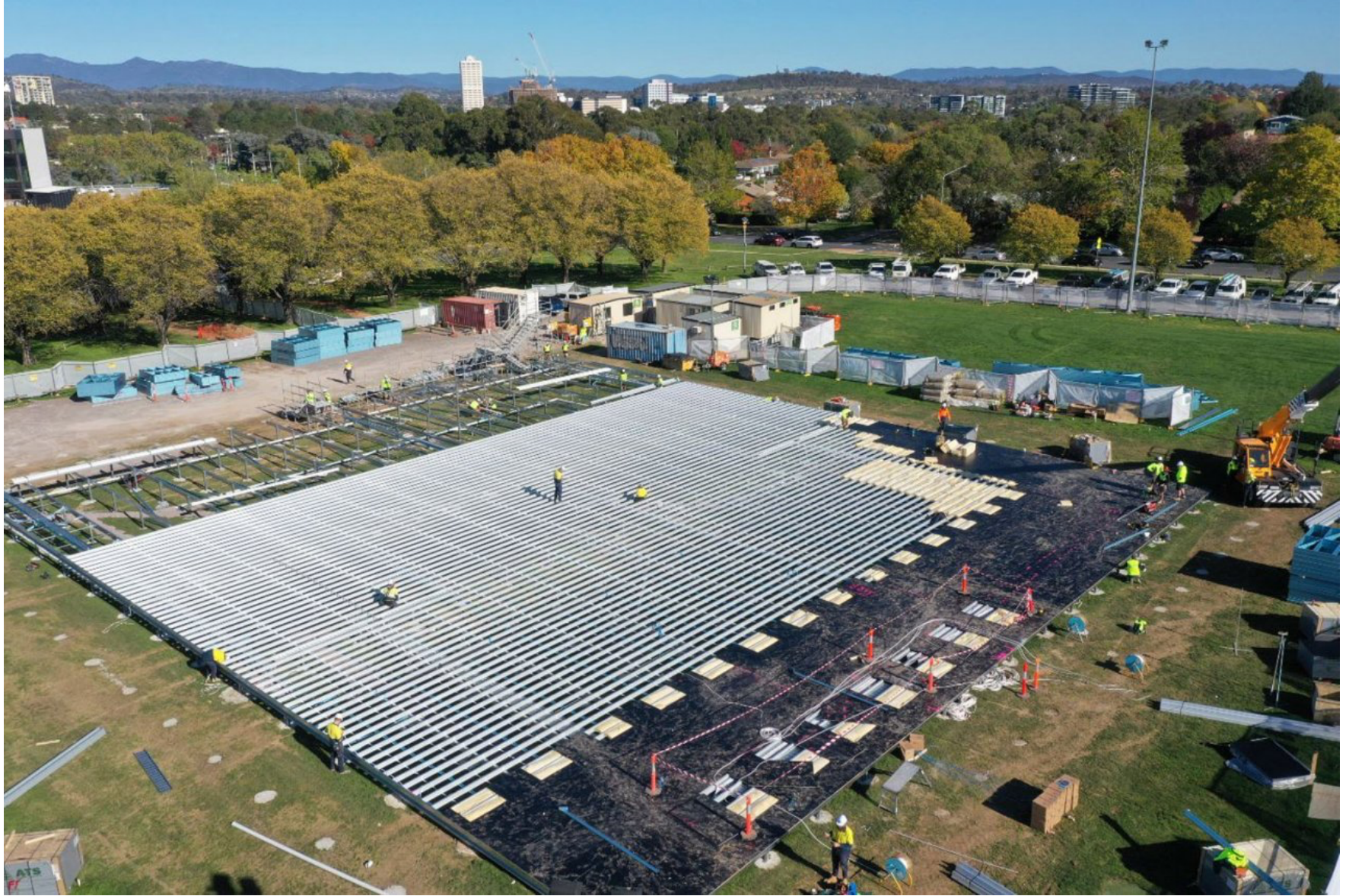
Site works of a medical facility developed by Aspen Medical in Canberra.
